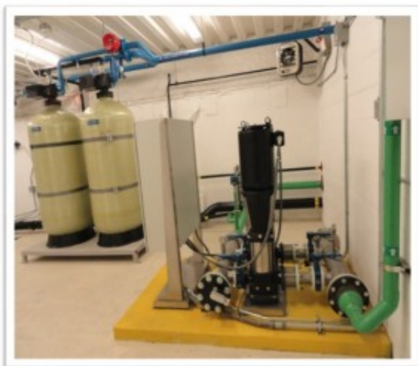
Nano-filtration water system
