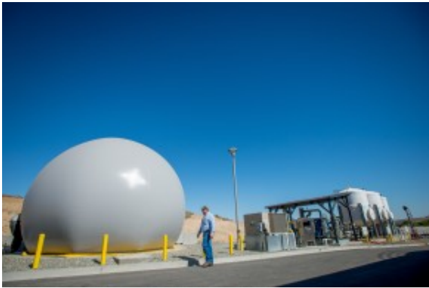
Biogas storage vessel
