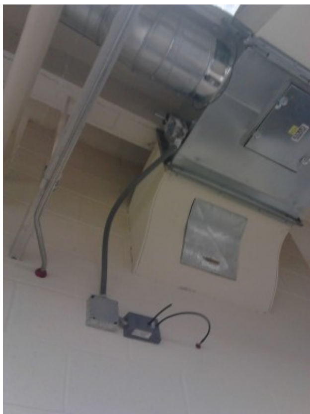
Upgraded ventilation system at a 3M lab
