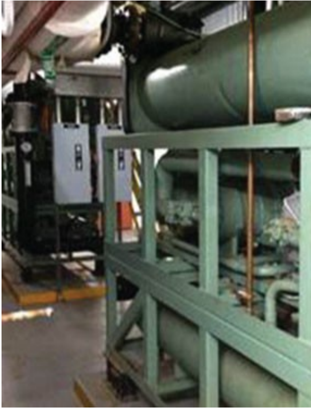
Two chillers to be replaced
