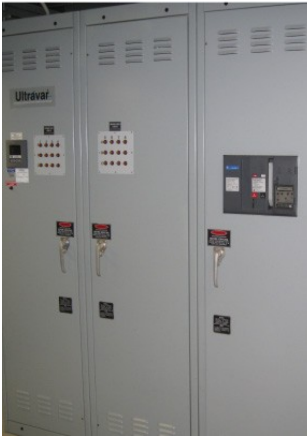
Capacitor bank improves power factor
