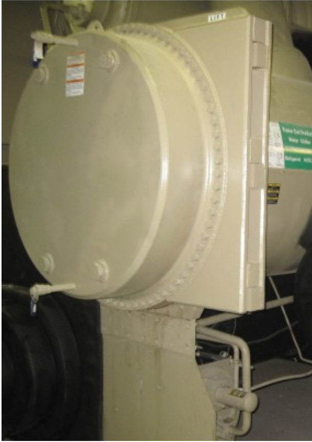
A newly installed chiller
